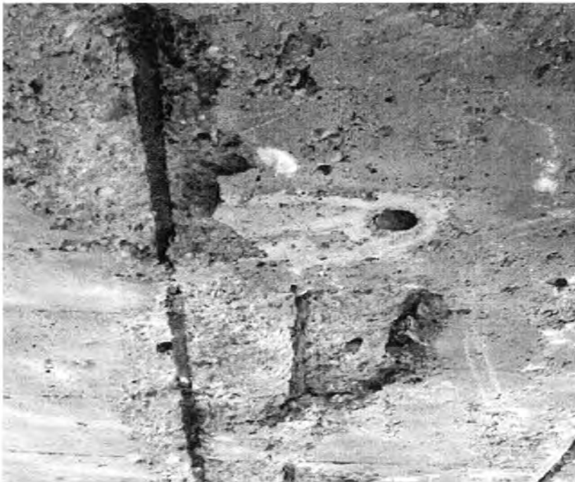
c. Reinforcing steel bars exposed on bottom of slab.
