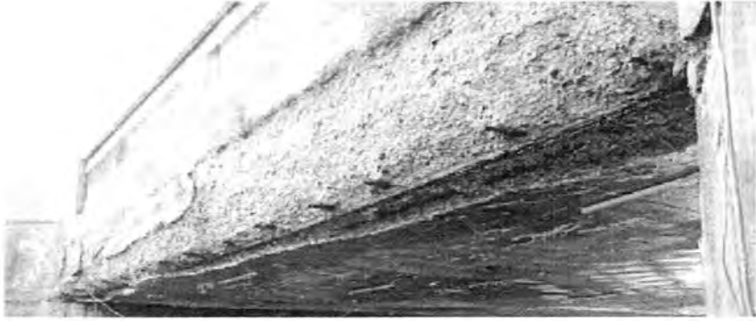
a. Spalling and heavy deterioration at edge.
